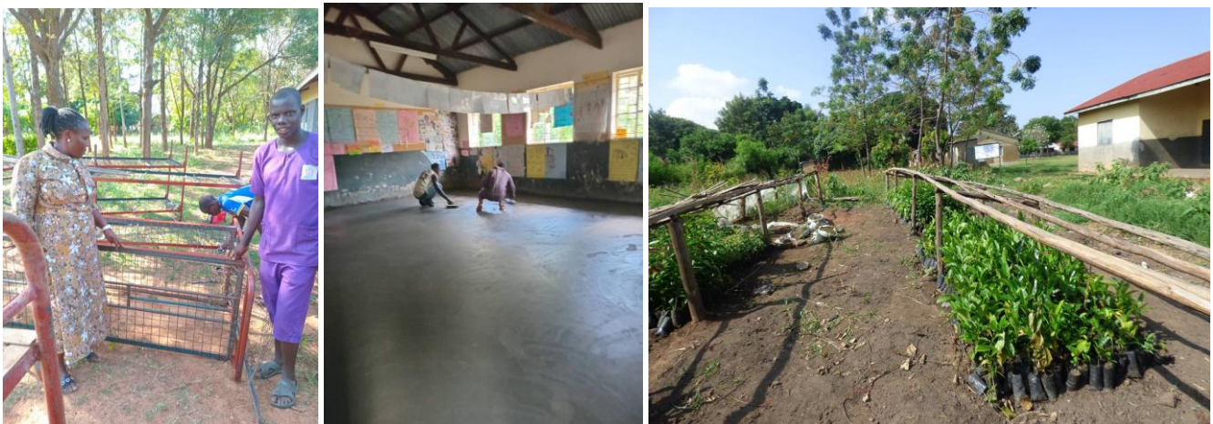
Stella with some of the repaired beds, floor work in progress and the tree nursery
